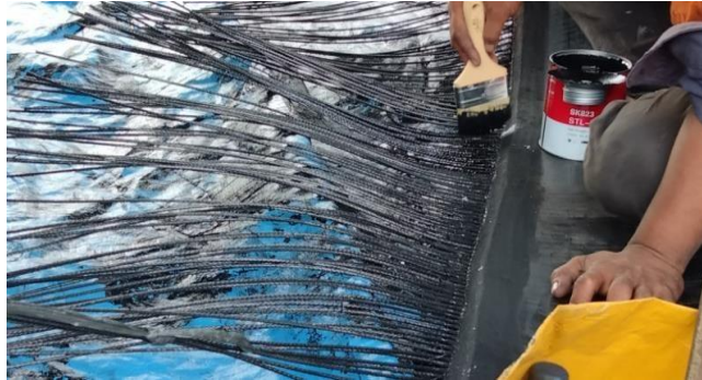
Gambar 8. Pengeleman Belt Conveyor
