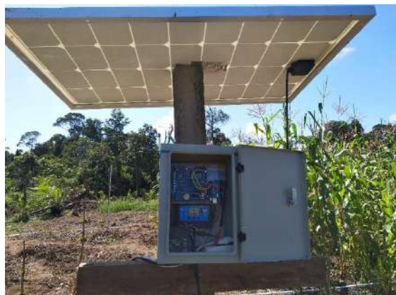
Gambar 5. Panel Sistem Kendali
